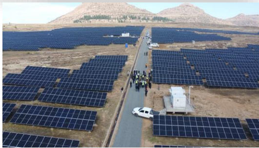
30MW Solar Plant commissioned 2023 - LEGCO
